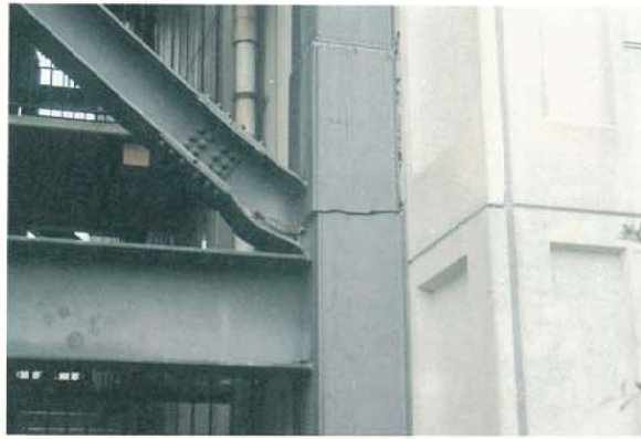
Photo 3.2.2.16 The fracture of vertical member with square-hollow-box section and H-shape brace.
