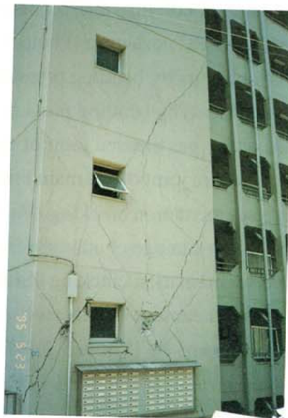
Photo. 3.2.1.15 Damage condition of the neighboring building (7 story frame structure; different one from the one of Photo. 3.2.1.14)
