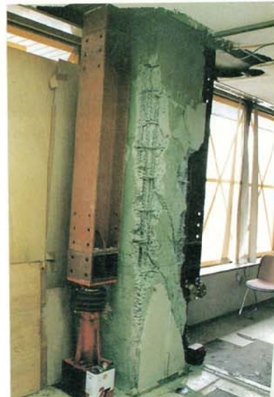
Photo . 3.2.1.62 Bond Splitting Failure of SRC Column
