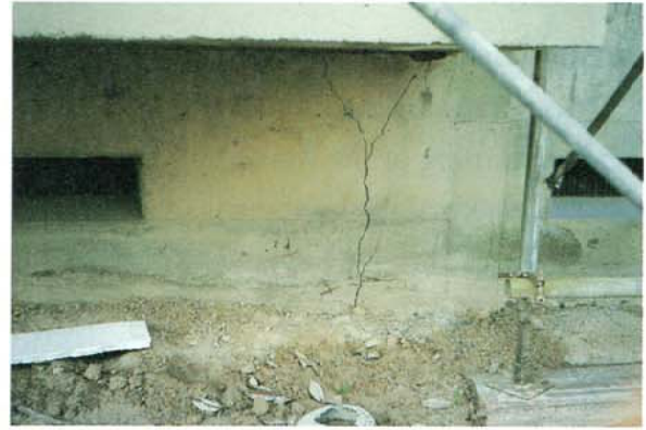
Photo. 3.2.1.13 Cracks of the base
