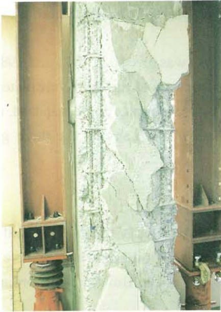
Photo. 3.2.1.39 Bond splitting failure of a column
