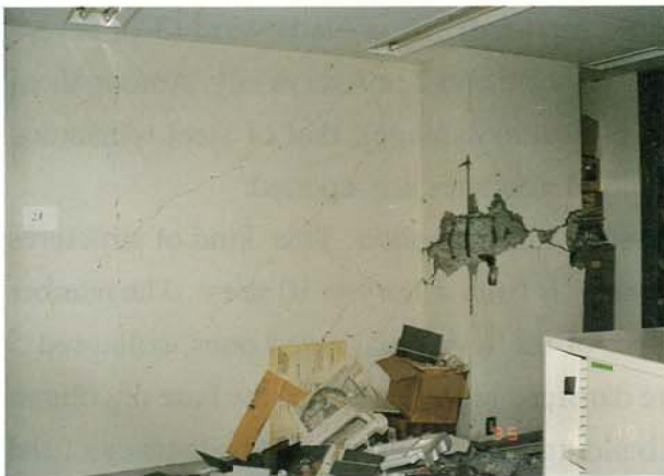
Photo.3.2.1.45 Bearing wall of the 2nd floor and the side column shear cracks ,buckling of the main column reinforcement
