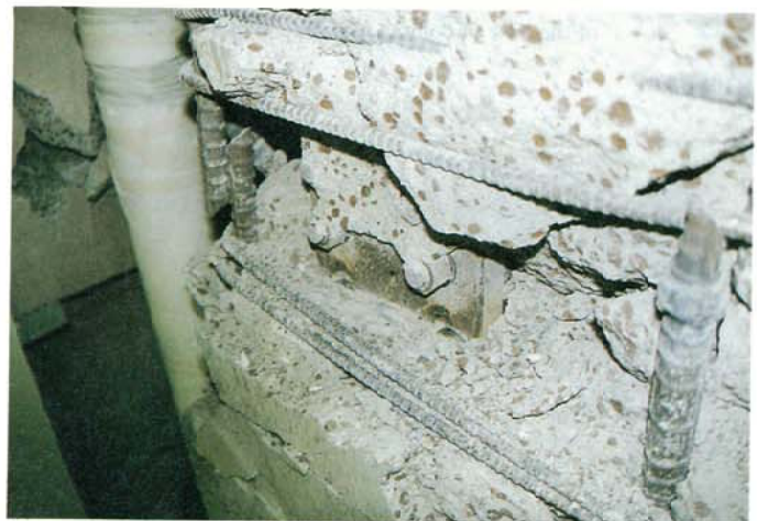
Photo. 3.2.1.6 11 story SRC structured governmental building Damage of the steel joint part of the peripheral column.(Fracture of the doubling plate of the joint part and the fracture of the main brace)
