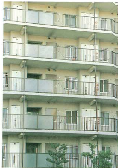
Photo . 3.2.1.66 Damage of Non-structural Partitions
