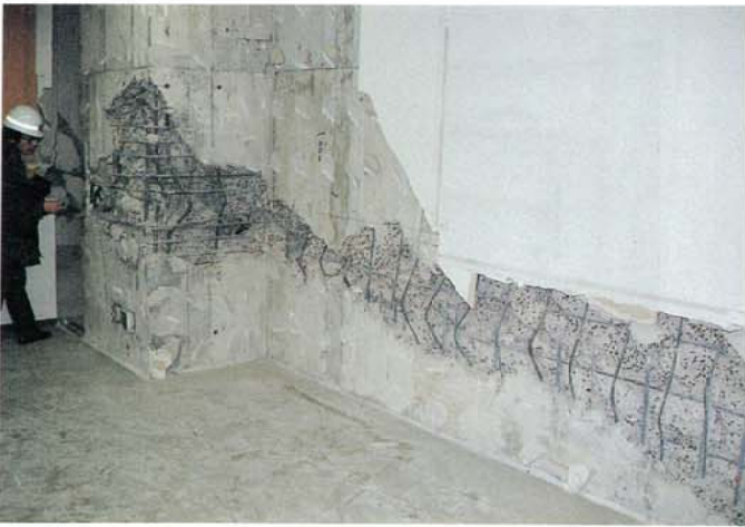
Photo. 3.2.1.7 11 story SRC structured governmental building Damage of the steel joint part of the peripheral column
