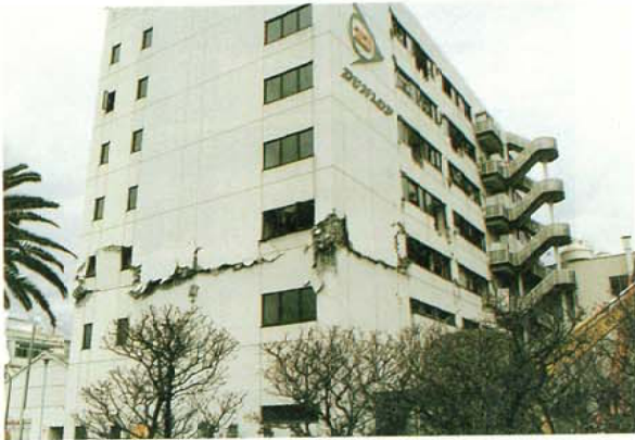
Photo . 3.2.1.60 Damage of relatively New Office Building
