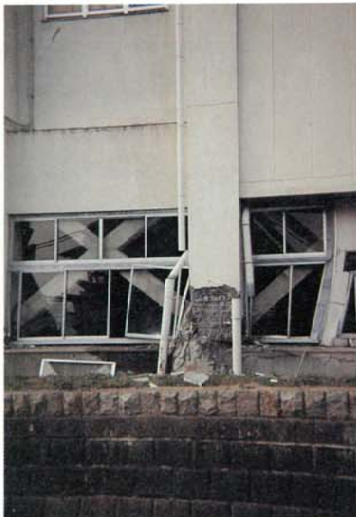
Photo. 3.2.1.8 4 story SRC structured office building The half of the column at the bottom of the anchor plate of the base of column was slipped to the north.
