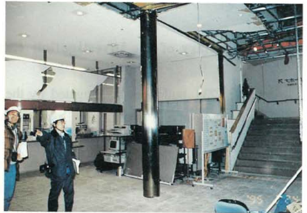
Photo 3.2.2.19 Damaged building interior due to pounding on parking building below (Building B)
