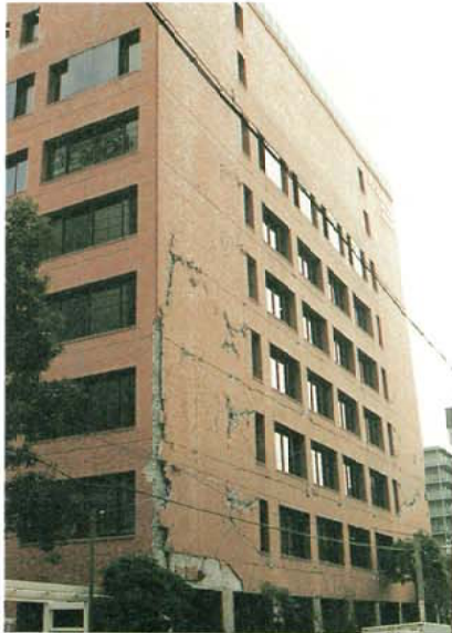
Photo . 3.2.1.65 Fracture of Anchor of Reinforcement
