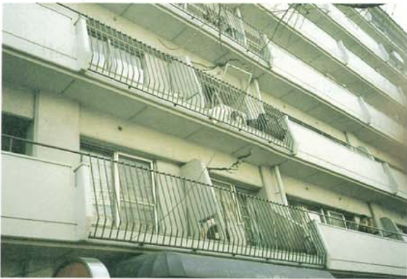
Photo. 3.2.1.41 Damage of beams mullion non-structural wall
