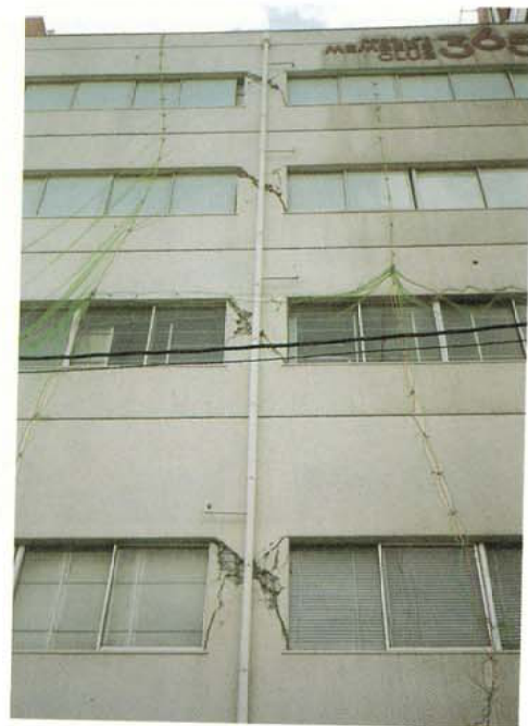
Photo. 3.2.1.30 Shear fractures of short columns
