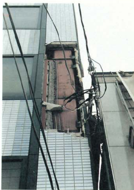
Photo 3.2.2.17 Two buildings collided.
