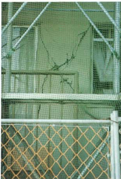
Photo. 3.2.1.12 Shear fracture creeping to the corners of the open part of the building ; windows & doors.
