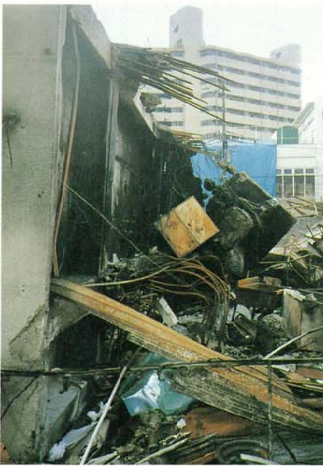
Photo. 3.2.1.18 Overturning of the whole building
