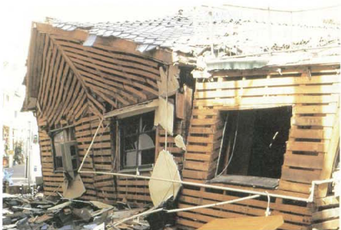
Photo 3.2.3.3 Collapse of the first story
