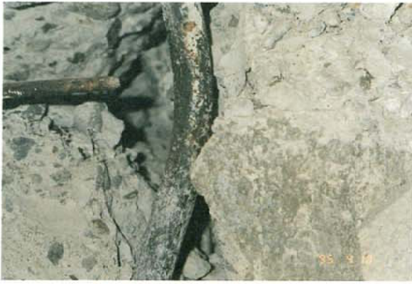
Photo.3.2.1.67 damaged hook by corrosion
