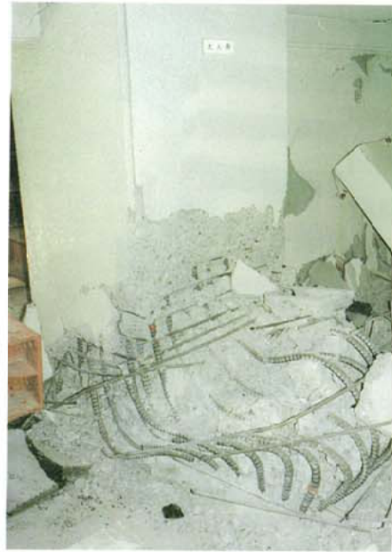
Photo. 3.2.1.56 Shear Crush of Column (1FL)
