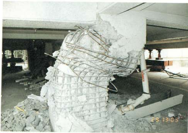
Photo. 3.2.1.31 Shear fracture of a column
