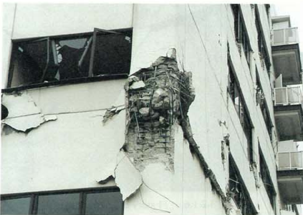
Photo.3.2.1.9 7 story (PH 1st floor) RC structured company building The shear fracture of the base of the column and the fracture of the foot of the earthquake resistant wall
