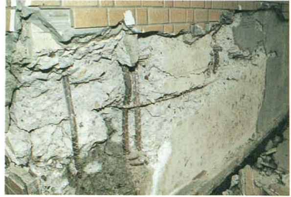
Photo . 3.2.1.64 Fracture of Splices of Steel
