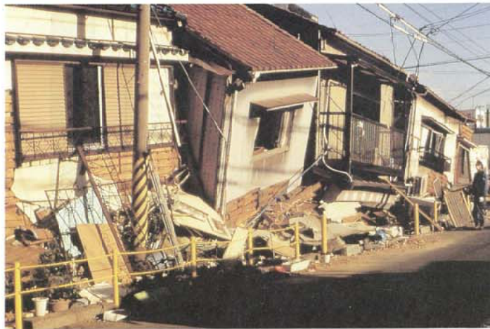
Photo 3.2.3.2 Collapse of the first story
