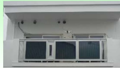
Test piece of solar hot water system for apartment houses
